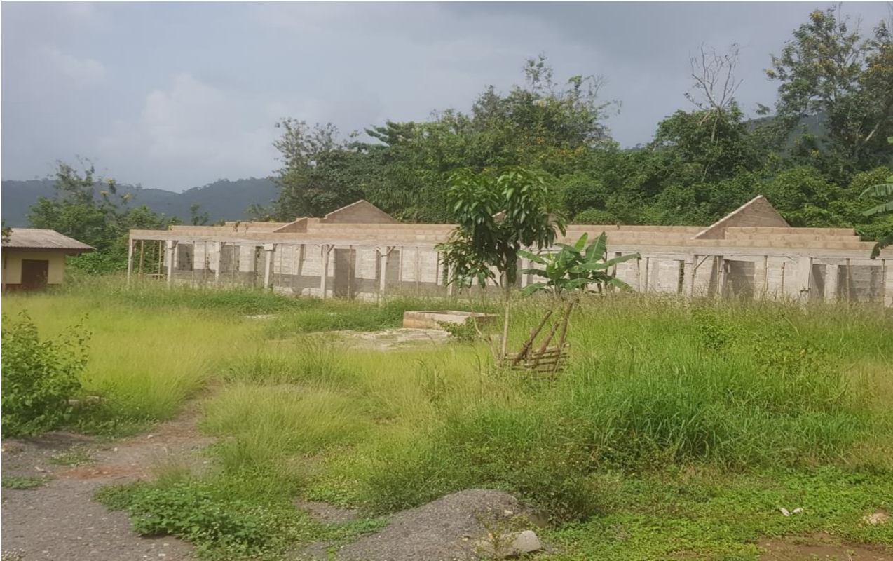
CONSTRUCTION OF 1 NO. 3-UNIT CLASSROOM BLOCK WITH OFFICE AND STORE AT OBAWALE – DACF-RFG (51% COMPLETED)
