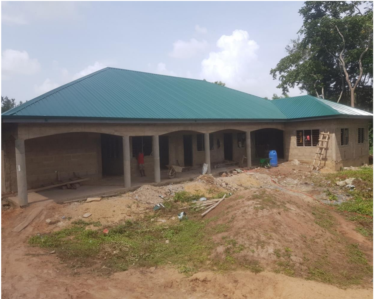
CONSTRUCTION OF CHPS COMPOUND WITH 1NO. MECHANIZED BOREHOLE AT AKETEBUOR – DACF-RFG (74% COMPLETED)
